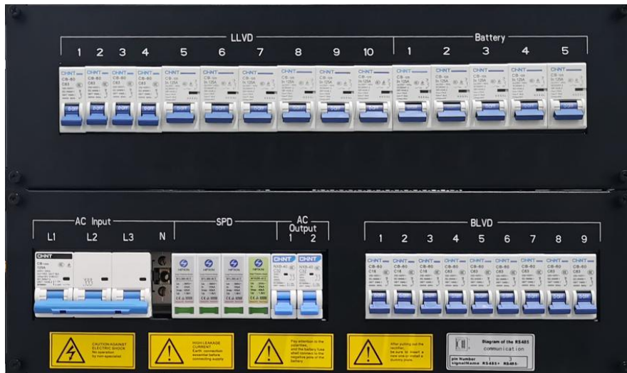
Figure2-4 AC/DC Power Distribution Unit
